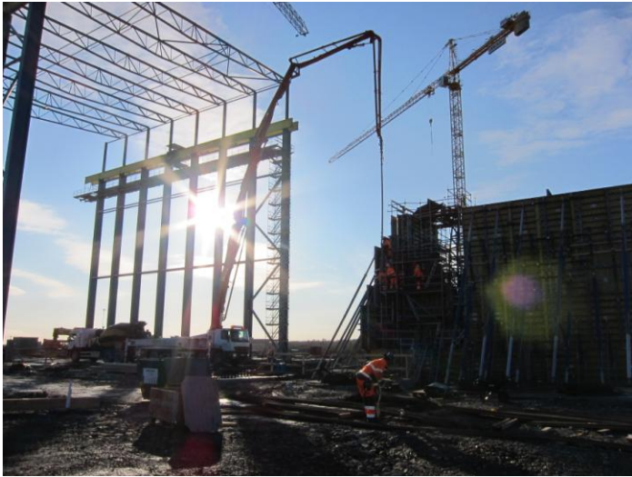
Construction of the Process Plant in Kaunisvaara. The steel works are currently being installed 24/7 on the site.
